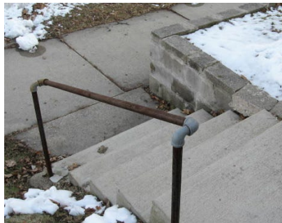
Pre-modification: Only 1 handrail on stairwell
