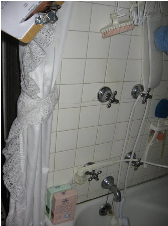
Image 4 Before: Shower with no grab bar to assist with transfers
