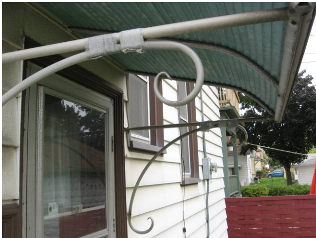
Image 8 Before: Awning taped together with duct tape
